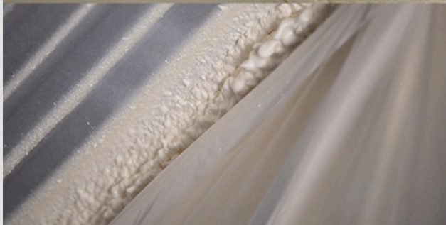
Two detailed views of the Polyurethane spray foam application proudly supplied by Pacific Urethanes.
